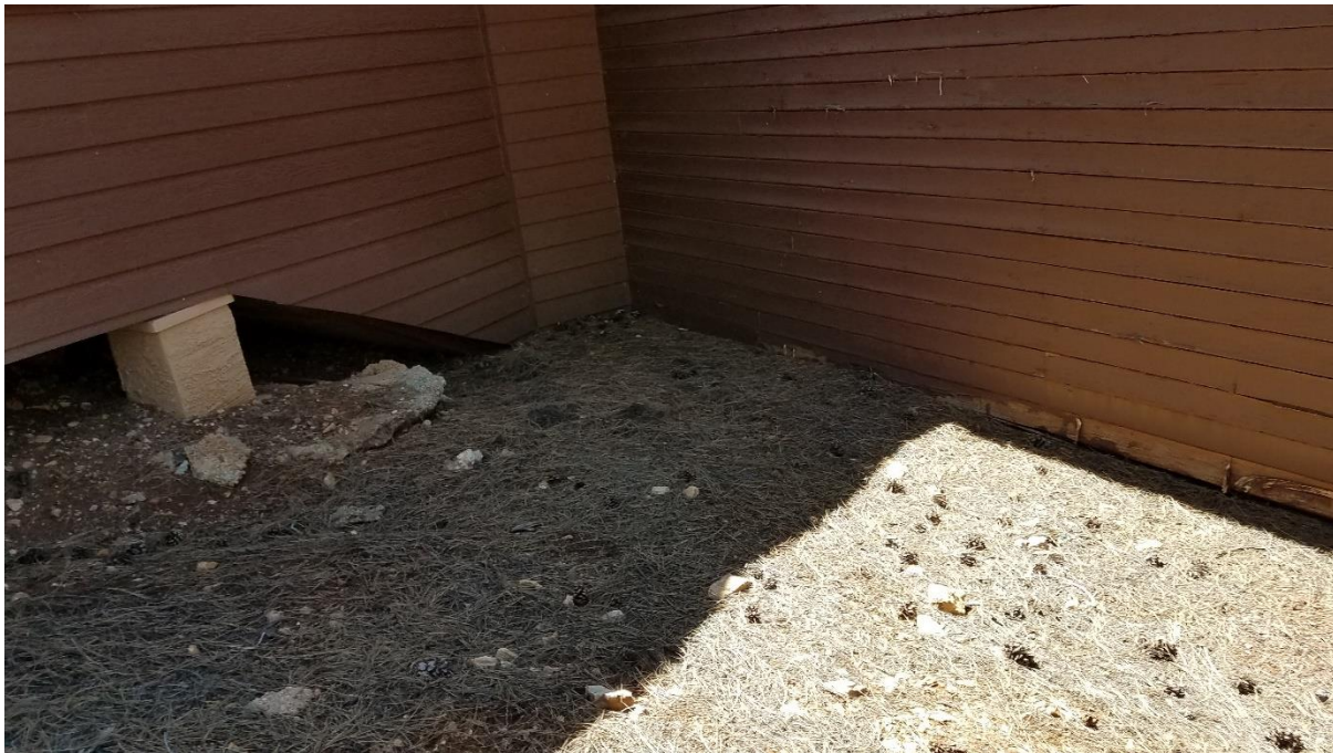
Figure 6: Example of surface flow causing erosion
